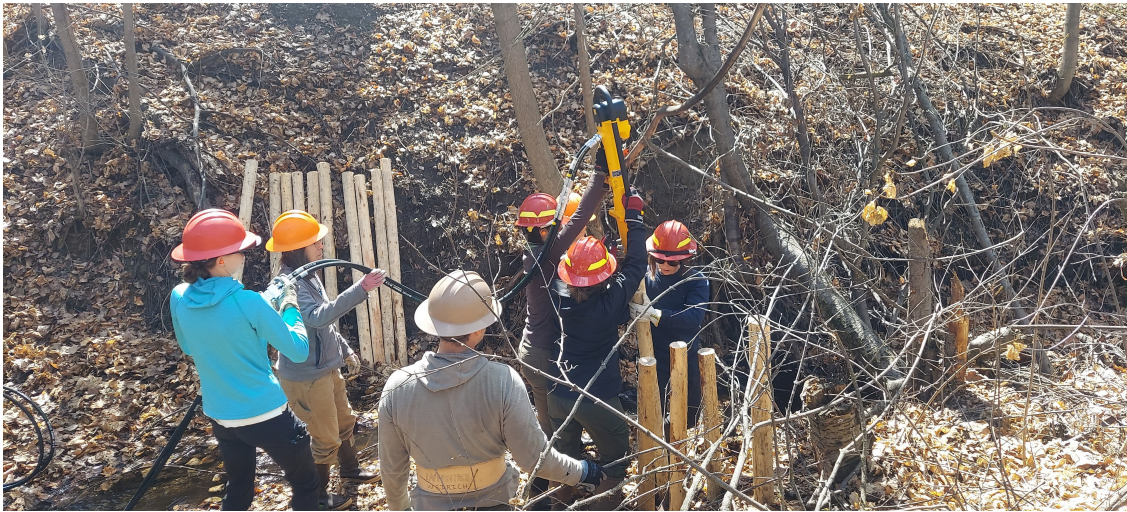
Installing posts for the beaver dam analog or BDA into the stream bed with our hydraulic post-pounder.
