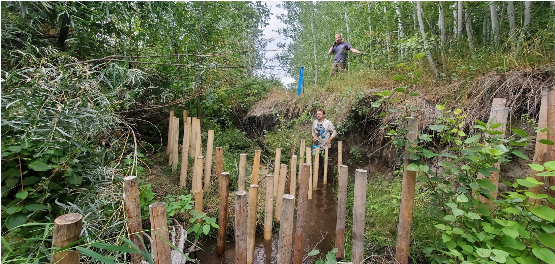
Above: Joe and Willy demonstrate the severe incision from post-wildfire erosion in this section of Chiliwist Creek.
