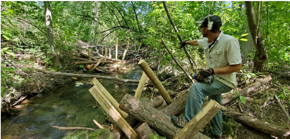
Structure Installation – July 2020 – intended to create channel sinuosity through erosion & deposition as well as push high flows onto the adjacent floodplains
