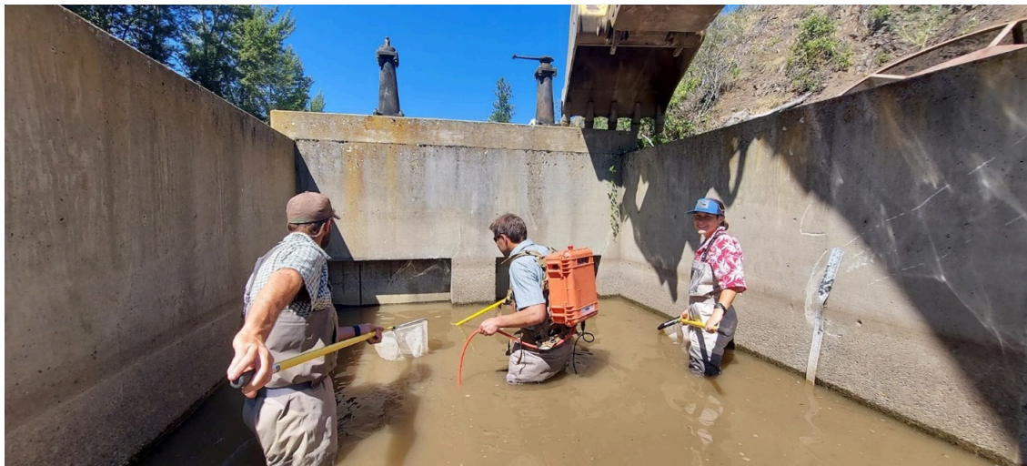
Katie helping relocate juvenile salmonids in July before a salmon habitat restoration project on a Methow River side channel that included removing the derelict concrete irrigation infrastructure seen in the photo.
