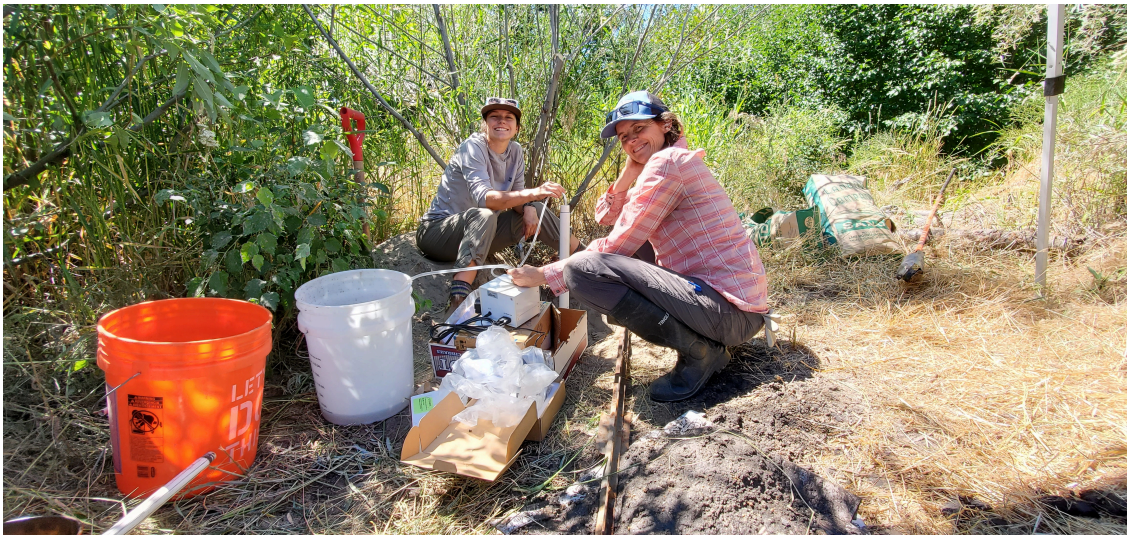
Installing & developing groundwater monitoring wells in Chiliwist Creek with MBP's Director and our fantastic 2022 summer intern from Colorado College.
